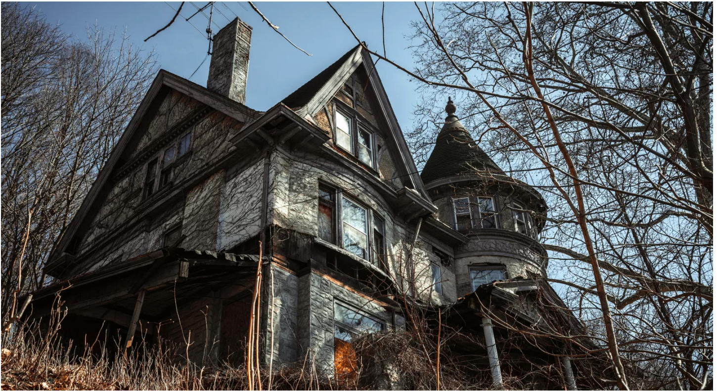
Mary Cardwell Dawson (left), and the deteriorating National Negro Opera House in Homewood.
